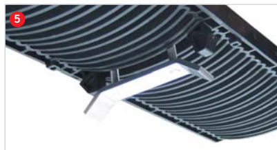
Fix the M6 security screws and clamp the grating as shown.
